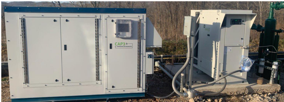
Figure 4. Field implementation of the CAP technology. On left is reach-in housing for compressed air storage. In middle is the 5650 Watt Stirling generator unit. On right is connection into a pneumatic controller structure
