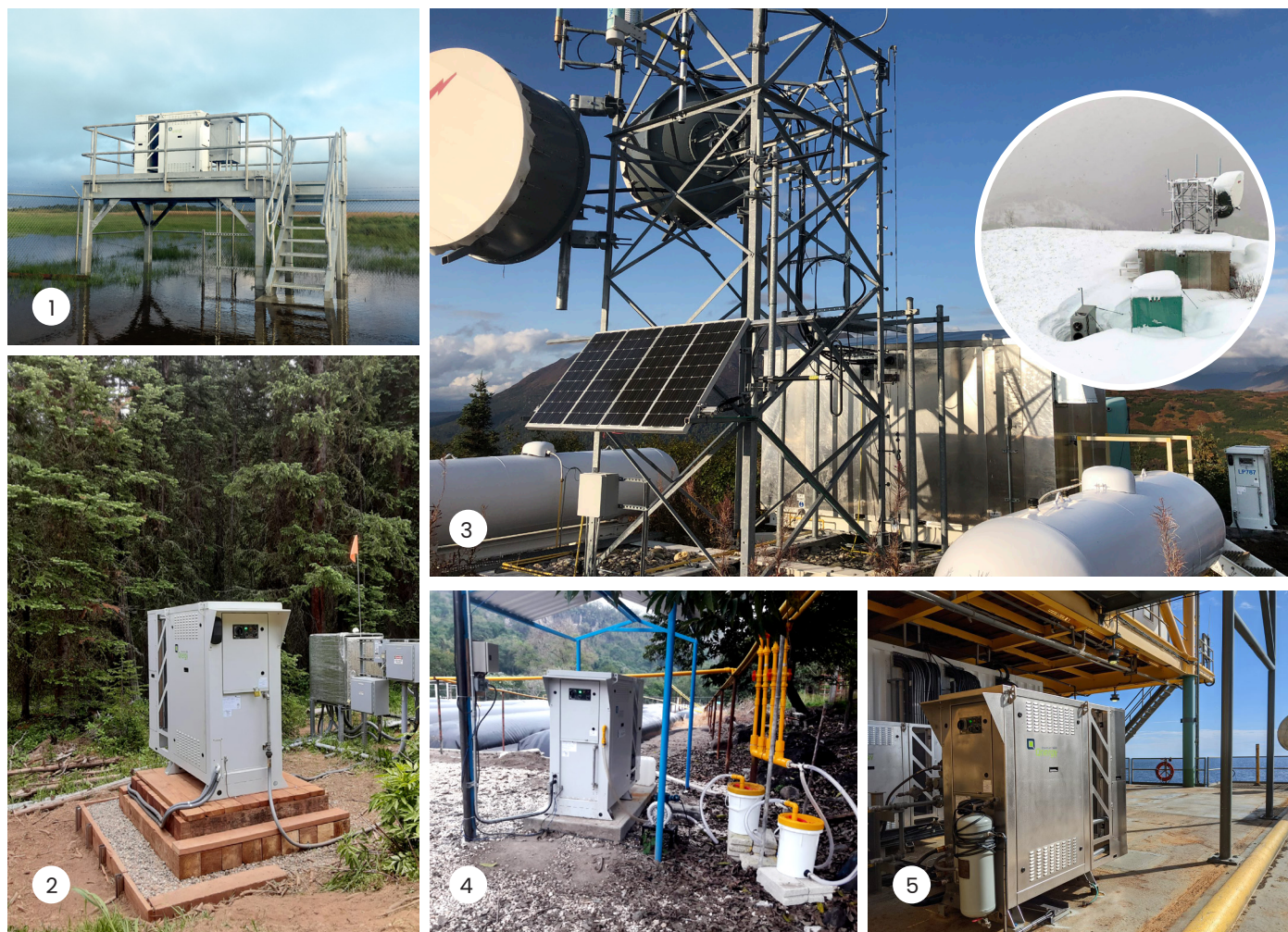
Figure 5. Qnergy's PowerGen platform in various installations working as both Prime and standby power. (1) A system in Louisiana supplying prime power for Cathodic Protection working after being through Hurricanes Laura and Delta; (2) A remote weather station in Colorado - Rocky Mountains; (3) Remote cell tower in Alaska. PowerGen on the right side of the picture serves as backup power for always-on telecommunication, charging standby batteries when needed using propane. The insert (circle, upper right) shows the system working during winter at -40F. This picture was taken through a helicopter window. Some of our distributed installations require a helicopter trip for maintenance. In those cases, the ROI of our elevated reliability is nearly immediate; (4) A pilot installation in Mexico in collaboration with Sistema bio utilizing biogas from animal manure digested in the sleeves in the left side of the picture. Low-pressure biogas is fed into PowerGen to create clean on-farm power; (5) Off-shore installation providing prime power to an unmanned platform in the Gulf of Mexico.
