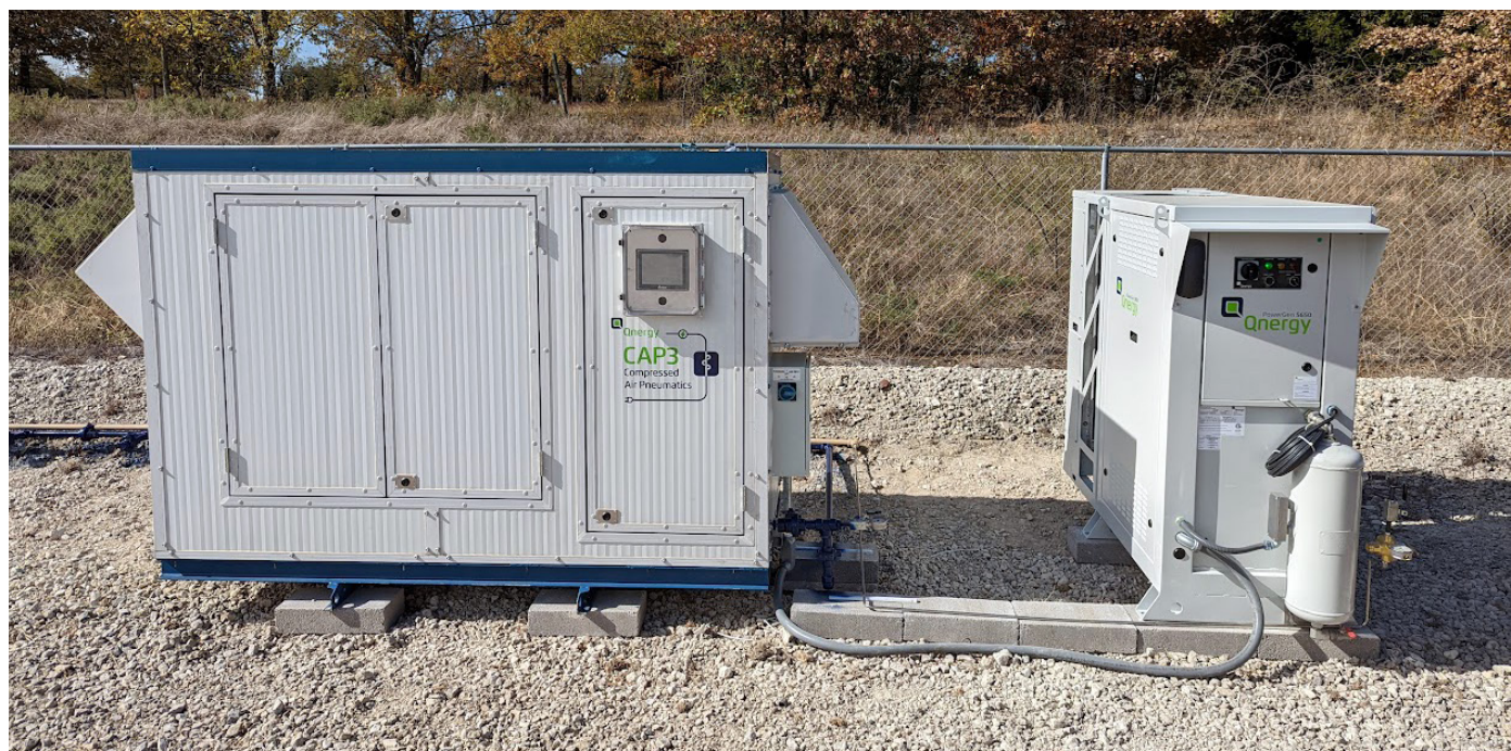
Figure 8. Qnergy CAP3™ system. Powergen 5650 engine/generator is depicted on right, the air compression system containing cabinet on left. Compressed air substitutes vented methane in powering and controlling pressure controlling pneumatic valves, eliminating vented methane. Hundreds of these units are deployed across North America to address the estimated millions of pneumatic controllers in use today.
