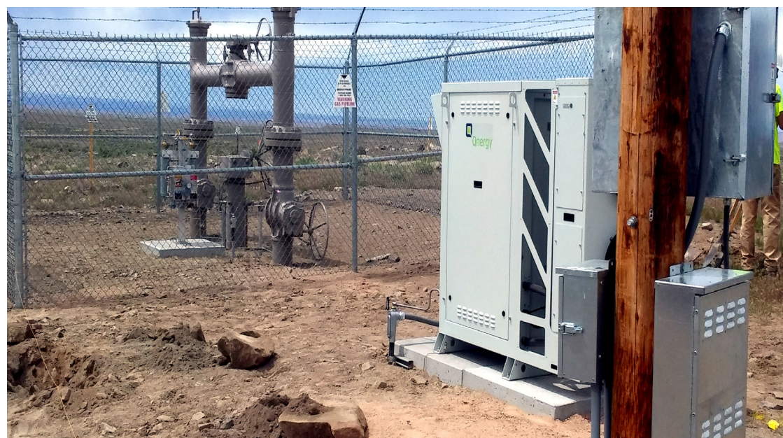
Figure 10. Qnergy PowerGen unit providing cathodic protection in the Colorado region. Unit is combined with a rectifier configured to match the power and direct current needs of the pipeline. Qnergy estimates that one such unit per 10 miles of pipeline is sufficient to provide protection against pipeline corrosion.
